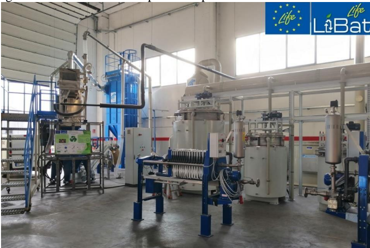
Figure 3. LIFE LiBat pilot plant overview
